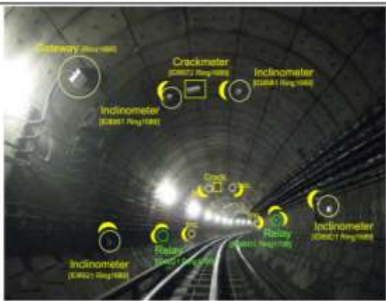
Figure 1. Wireless sensors locations in a tunnel by Prof. Kenichi Soga Professor of Civil Engineering Department of Engineering [10].
