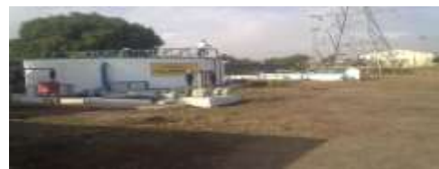
Fig.no. Primary clarifier
