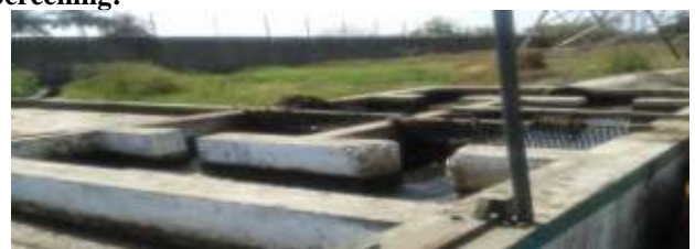
Fig. Screening chamber
